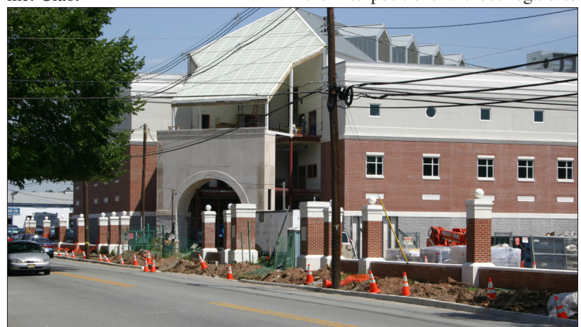
Benjamin B. Corbin for The Westfield Leader and The Times TAKING SHAPE...The modern Union County Police Headquarters under construction on North Avenue in Westfield is rapidly taking shape. The new center is one of the largest structures in the town and merges with the other county buildings on the avenue in providing a bustling government service center.
